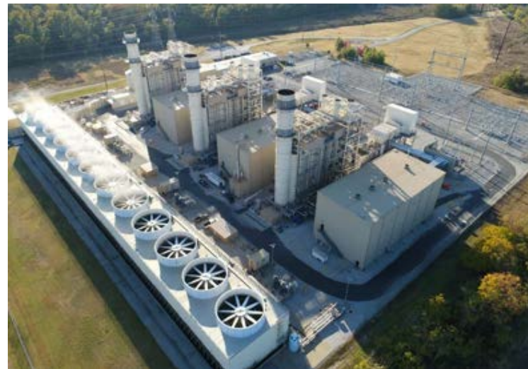
Green Country Natural Gas Plant 795MW CCGT, Jenks, OK – Photo Credit, www.psoklahoma.com
